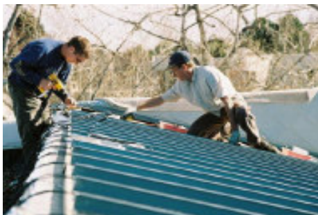
Thin-Film Solar on a Metal Roof
